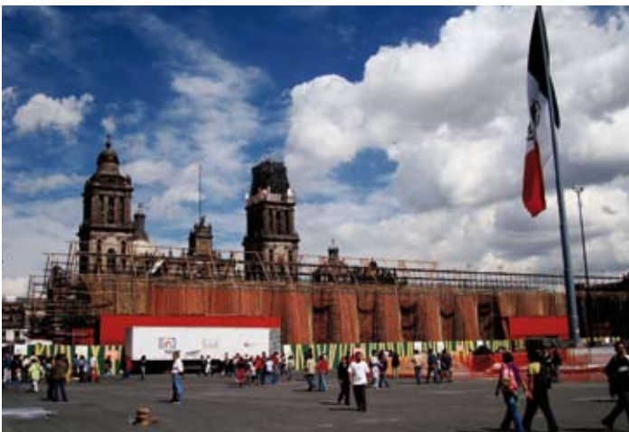
El nomadic museum, Mexico City, place de la constitution, en 2008, en cours de montage. / Constitution Square, in 2008. During construction.
